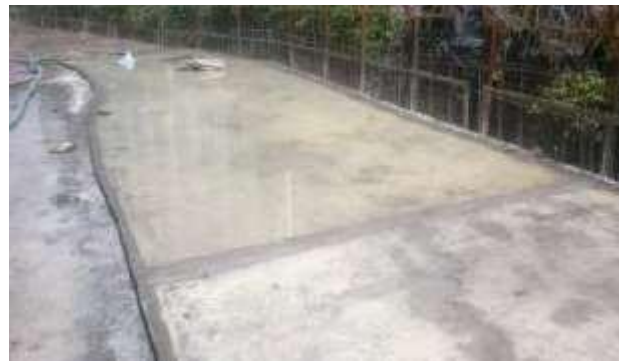
Fig:16 Ponding of slab
